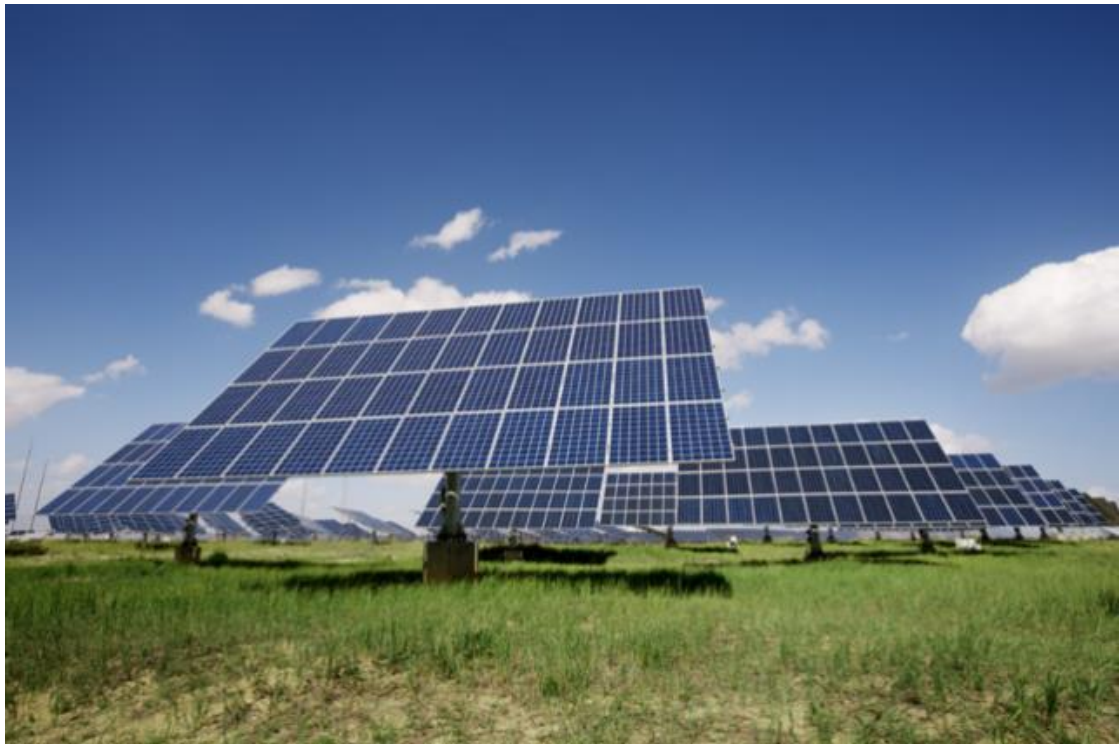
A corner of the 100 MW Demonstration Power Station
